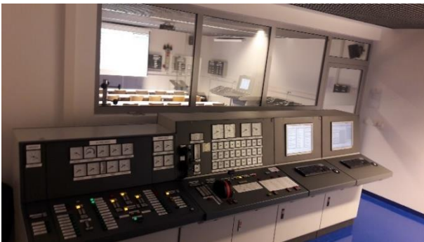
Figure 4: Kongsberg Simulator Control Room
